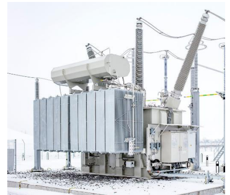
Transformers & Shunt Reactors
