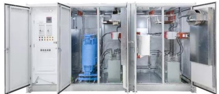
MV Capacitors & Filter Bank
